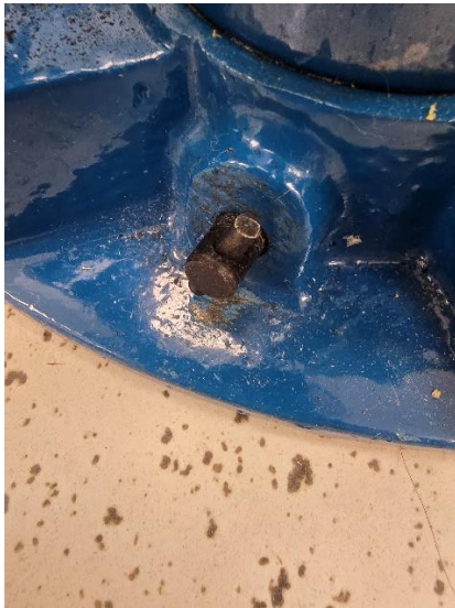
Figure 275: Closeup of Release Valve
